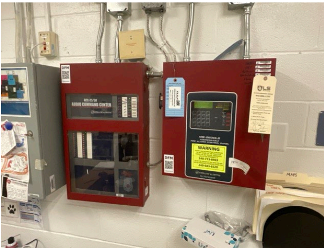
15 - FIRE ALARM PANEL
